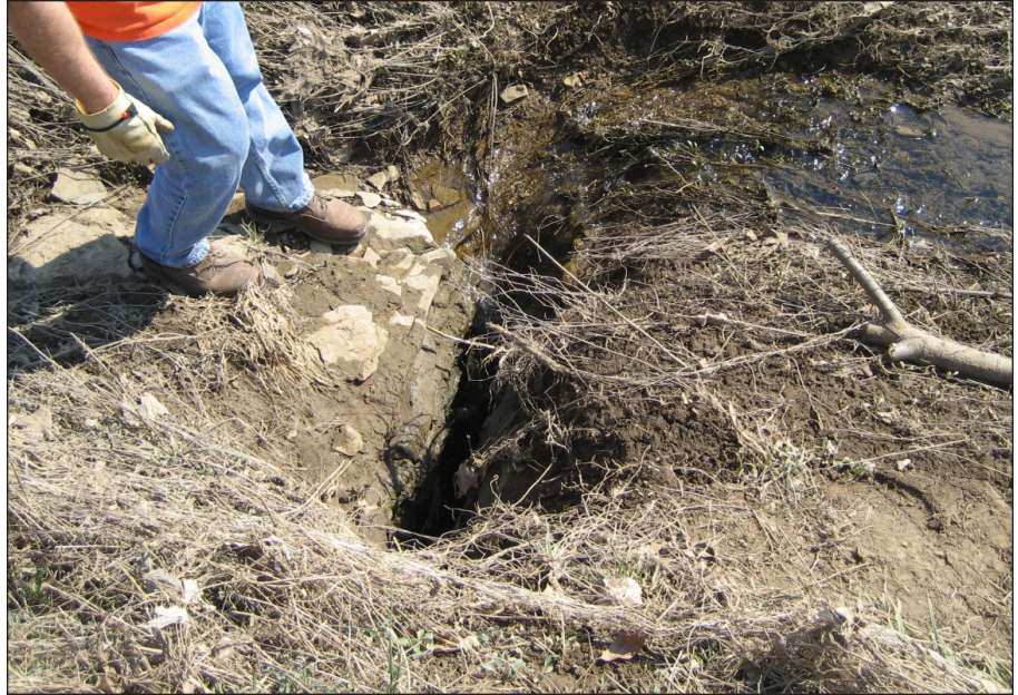
Figure 1. Flow from a small stream enters into the ground by way of a large swallow hole.
