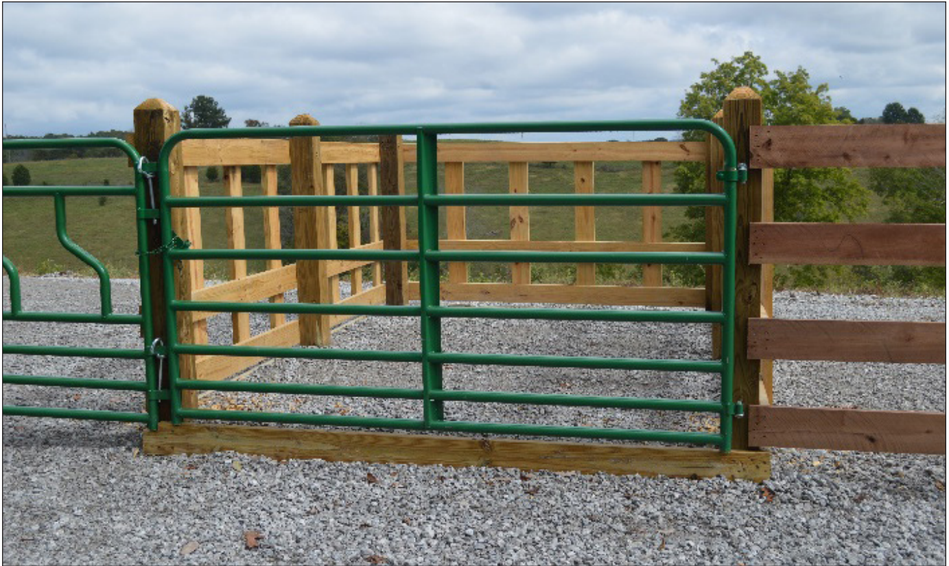
Option 4. Uncovered structure with wood panels and geotextile fabric and gravel pad surrounding.
