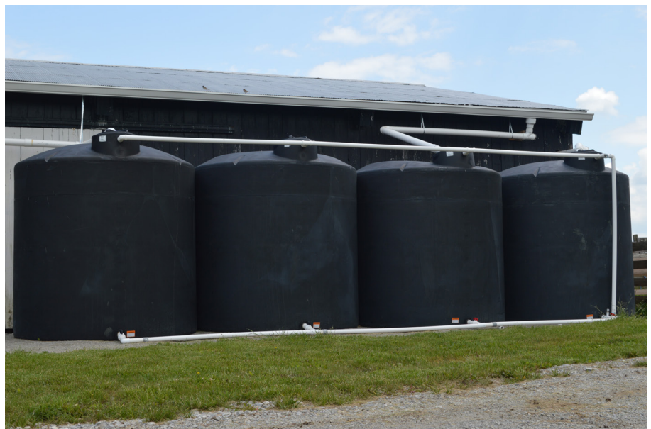
Figure 3. A series of aboveground tanks that have been connected together to create one large storage system. Valves on the pipes coming out of the bottom of each tank allow tanks to be drained and managed individually, if necessary. A common overflow pipe plumbs overflow water from the tanks outside of the production area. Similar concepts may be applied to cisterns. Photo by Lee Moser
