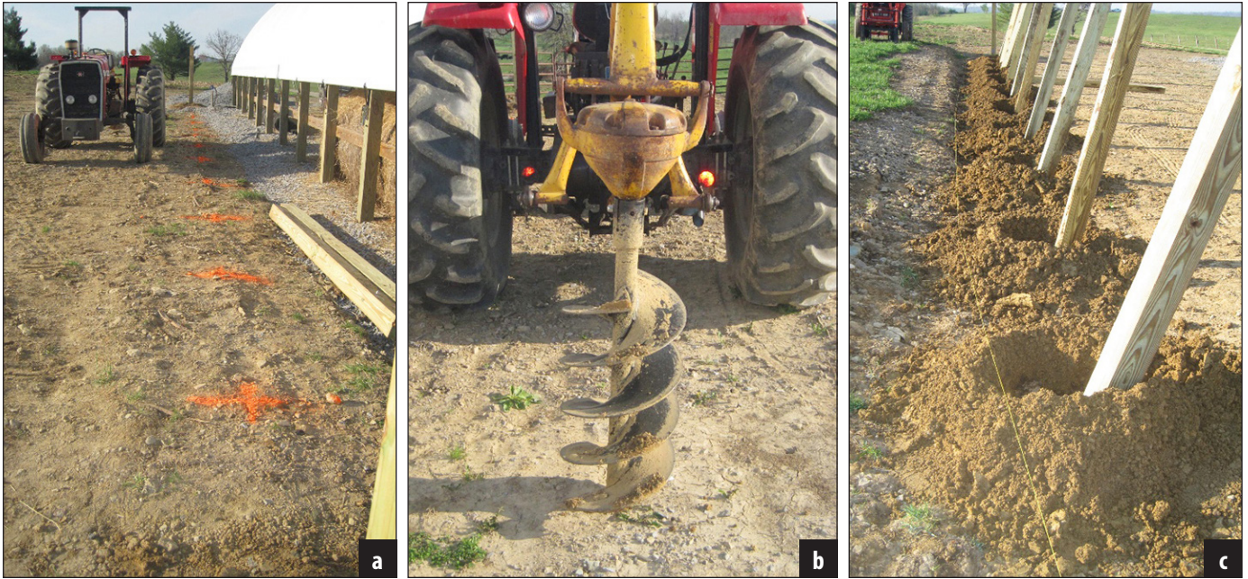
Figure 4. Mark locations for the posts along the sidewall. Dig the holes with an auger. Place the posts in the holes.
