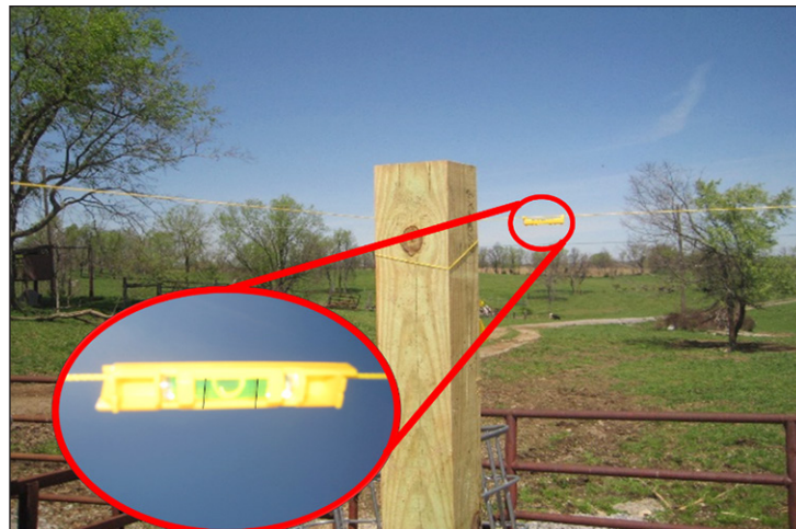
Figure 7. The string line provides a way to visualize the height of the knee wall.
