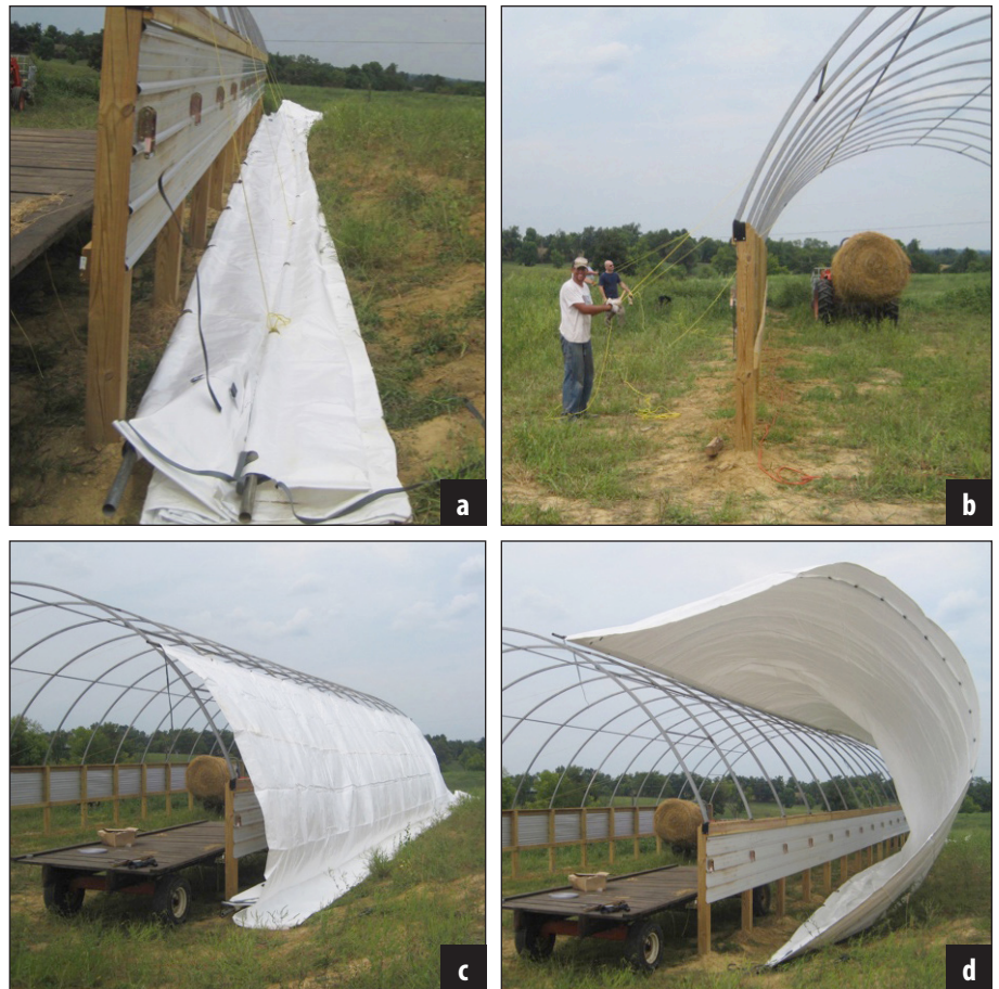
Figure 19. Setting up the nylon ropes to pull the tarp and pulling it into position.
