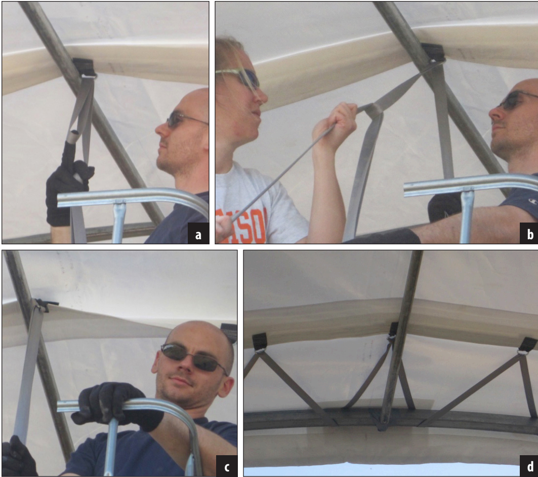
Figure 23. Beginning to lace the tarp along the end starting from the center at the top of the hoop.
