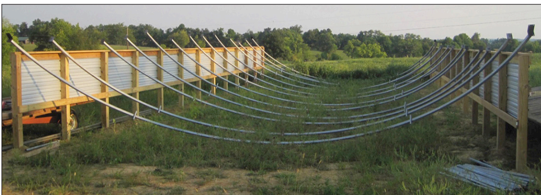
Figure 12. The ribs are set up in preparation for raising them above the knee wall.
