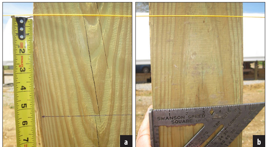
Figure 8. Measure down from the string line. Mark the bottom line using a speed square.
