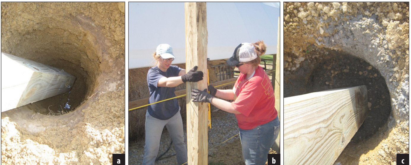
Figure 5. Anchor the posts with prepared concrete. Ensure that the posts are upright and properly spaced. Backfill the post hole with soil.
