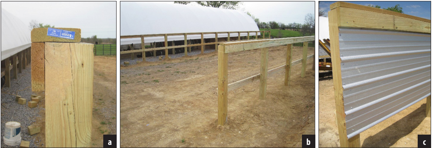
Figure 10. Treated 2 x 6 inch 12-foot-long fence boards are placed on the top of the knee wall and 36 inches up in the inside of the sidewall and screwed into each post. One run of metal siding was placed along each sidewall.
