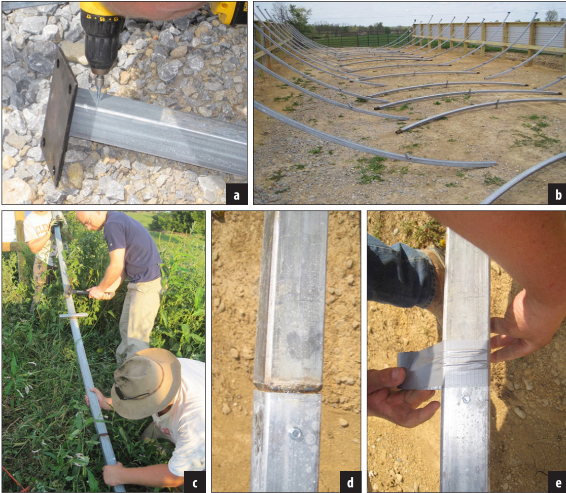
Figure 11. The construction of the ribs, including attaching feet, setting up the ribs, and connecting the rib sections.
