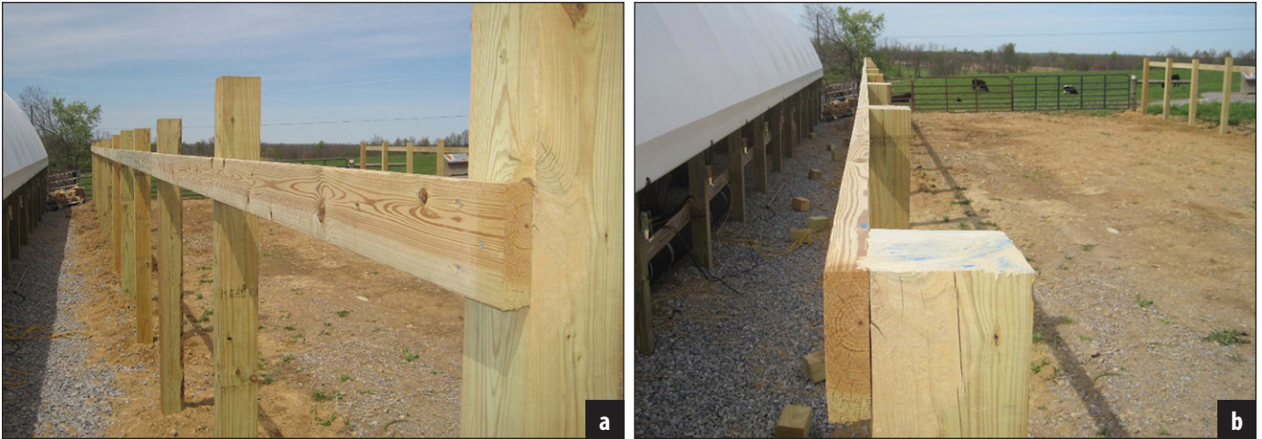
Figure 9. Treated 2 x 6 12-foot-long fence boards are placed above the marked line on the post and screwed into each post. The fence posts are cut off at the top of the 2 x 6.
