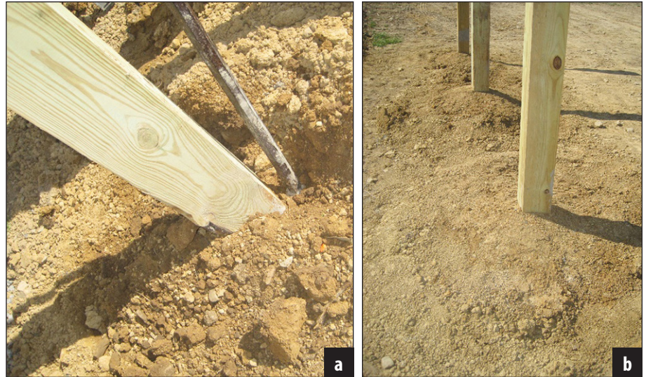
Figure 6. Tamp the soil down with a digging iron. Mound the dirt around the post for extra stability and to divert water away from the post.
