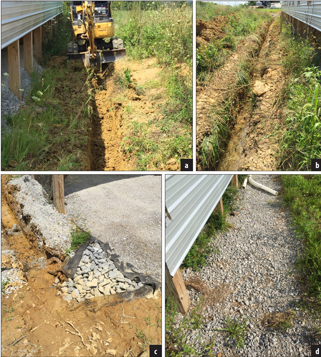
Figure 28. Creating drainage along the sides of the hoop barns. Ditches include large rock surrounded by filter fabric and covered with smaller rock.
