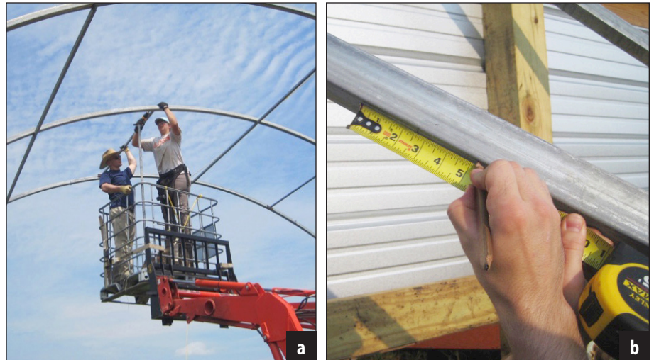
Figure 16. Adding additional cross bracing between the outside two ribs and marking these locations on the ribs.
