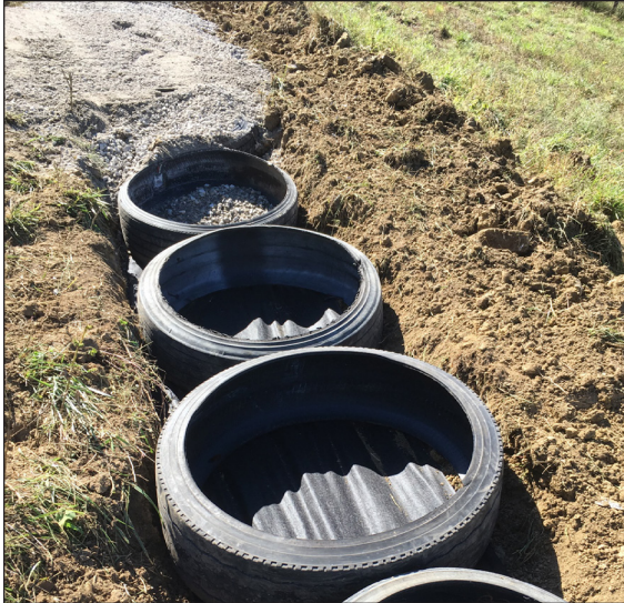
Figure 4. Nonwoven geotextile fabric and tread cylinders are placed in a trench and backfilled with dense-grade aggregate (DGA).
