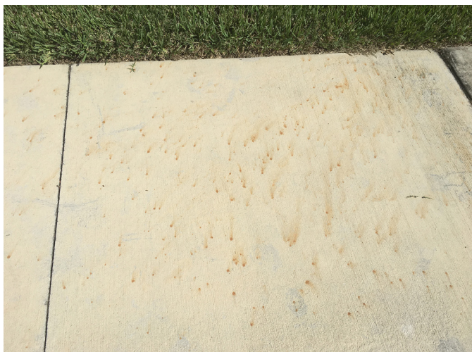
Figure 3. Granular iron sulfate fertilizer particles will rapidly dissolve and stain wet surfaces such as this sidewalk.
