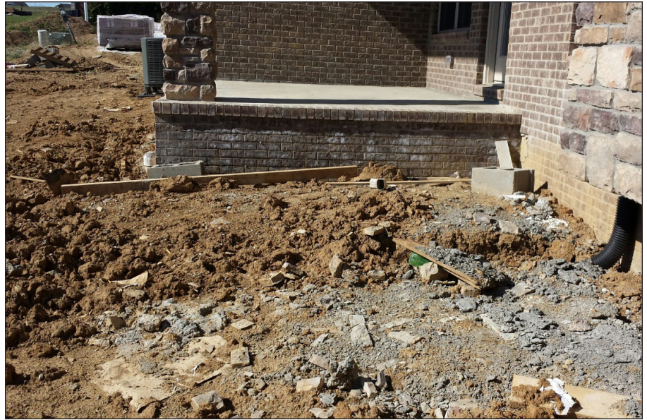
Figure 2. Building debris remaining around foundation of house following construction. If buried, this debris will cause difficulties in growing a lawn or landscape plants.
