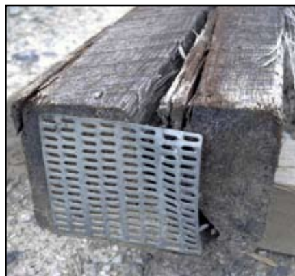
Figure 30. End plates can't salvage every tie.
