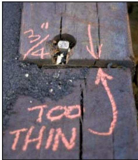
Figure 34. One of these crossing ties is obviously not the right thickness!
