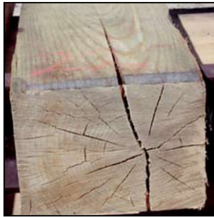
Figure 27. This split is acceptable as-is for an air-dry tie. It is less than \frac{1}{4} " wide and shorter than the 9" face where it appears. (Remember that the tie end doesn't count as a surface.)
