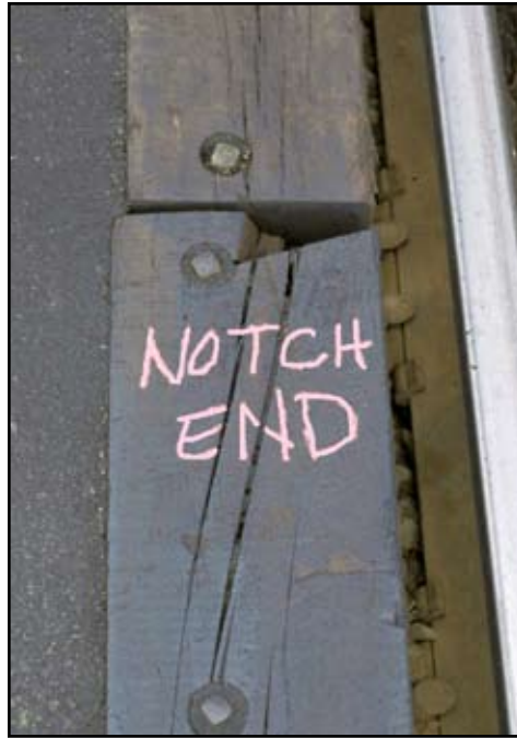
Figure 33. The miscut end should have caused this tie to be culled. This cut is from the felling notch in the woods.
