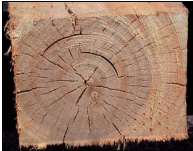
Figure 23. The combined width of these two ring shakes is 4", which causes rejection under a 9" face width.
