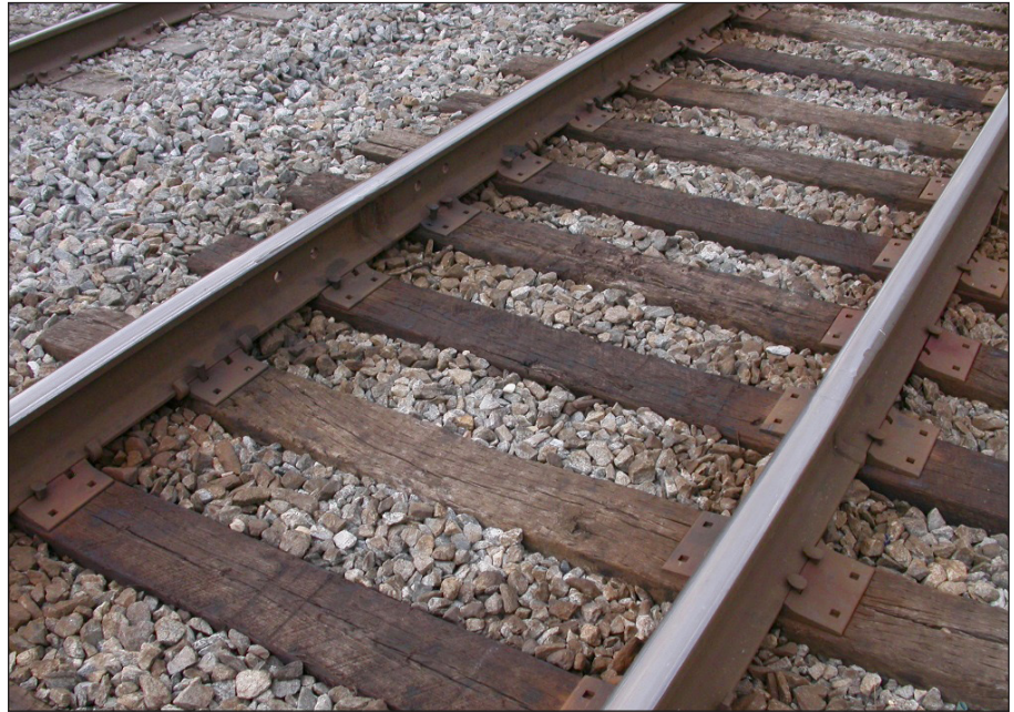
Figure 1. Section of railroad track used to move freight through Lexington, Kentucky. This track uses wooden crossties.
