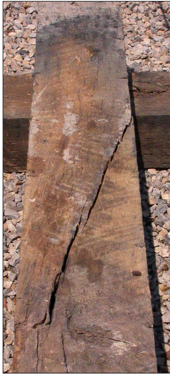
Figure 13. This tie was culled for slope of grain.
