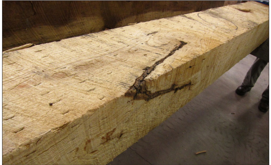
Figure 15. Bark seam in a tie due to a branch.
