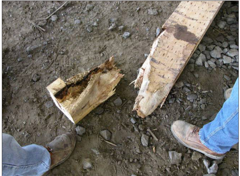
Figure 14. This tie broke when I picked it up. There was a combination of slope of grain and decay here.
