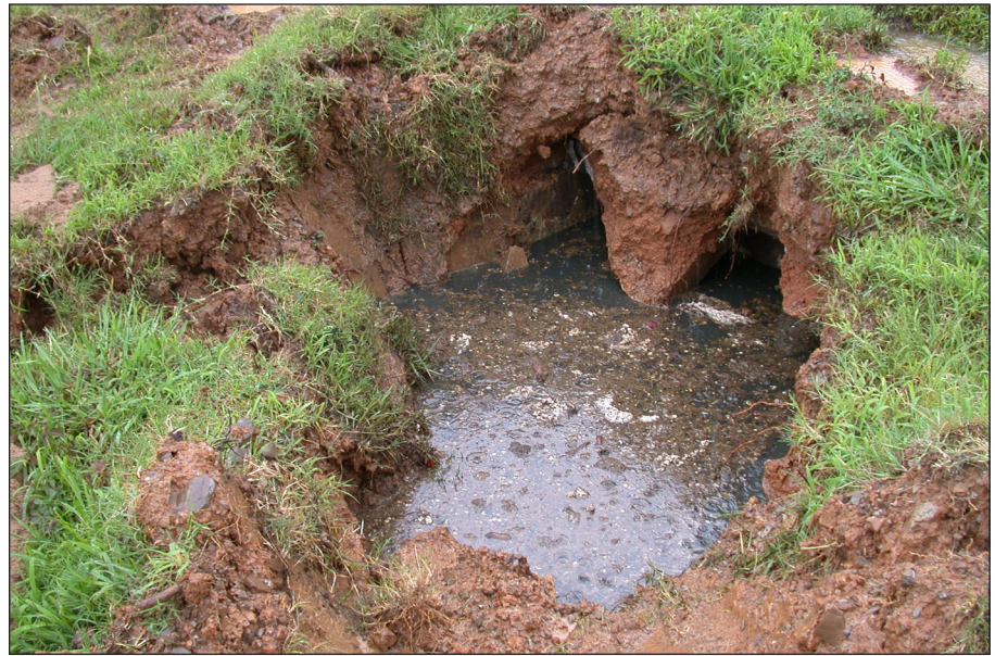
Figure 4. Photograph of a concrete septic tank lid that has collapsed under a truck's weight. Repair costs were more than $1,000.
