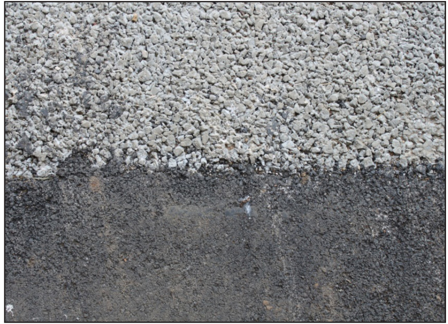
Figure 3. Pervious pavement (upper portion) offers a number of environmental benefits as compared to standard asphalt (lower portion).
