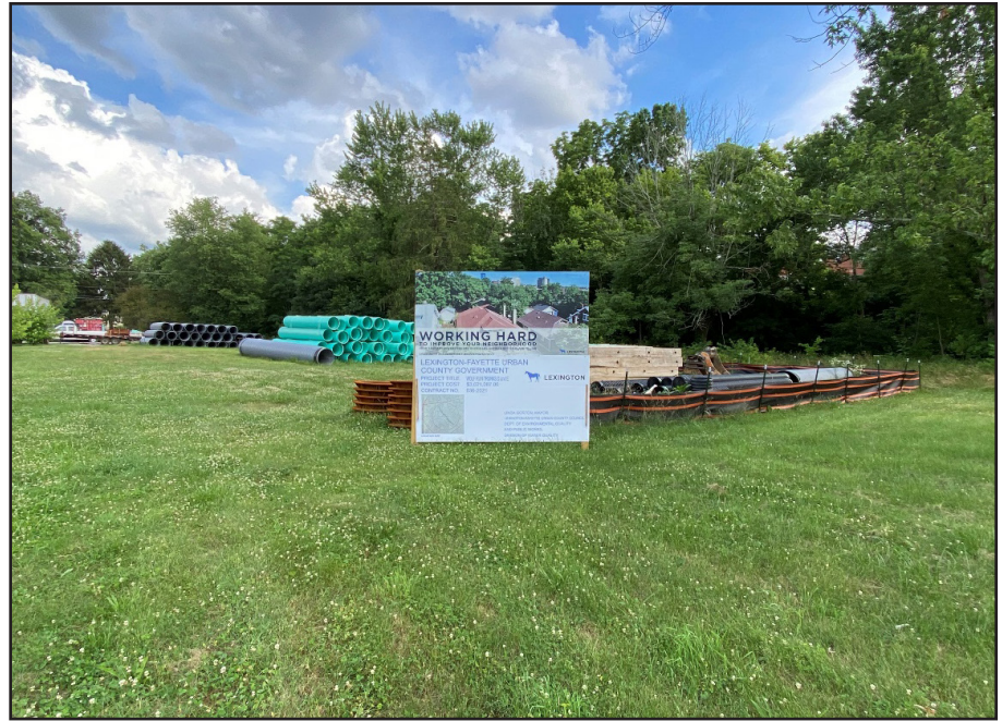
Figure 3. A staging yard for a sewer line replacement project in the Wolf Run Watershed.
