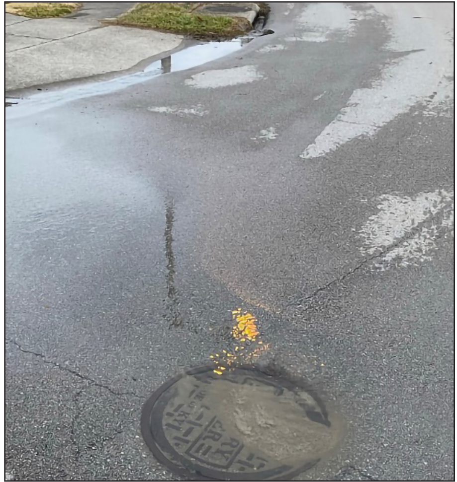
Figure 1. A sanitary sewer manhole in a separate system overflowing into a nearby storm sewer that discharges directly to a local waterway.
