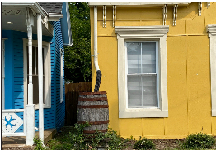
A rain barrel used for residential rainwater harvesting. Photo by: Lee Moser
