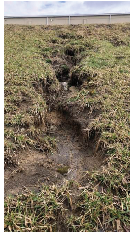
Concentrated stormwater flow has eroded sediment from the embankment, forming a gully.
