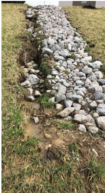
Stormwater erosion has formed a gully on the left side of the forebay.
