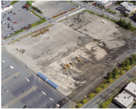
Figure 10. Before, during (below), and after (far right) construction of the Thornton Creek water quality channel. SvR Design Company 2009
