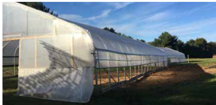
Figure 12.4 Windstorm-shifted tunnel. Windstorms moved tunnels when anchors had not been fully installed. Note the structure has been picked up and moved diagonally in the plot.
