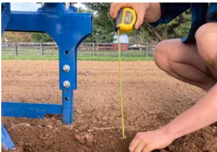
Figure 49. A worker checks the depth of the drip lines being installed with the Andros drip layer.
