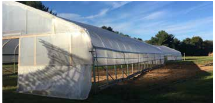
Figure 12.4 Windstorm-shifted tunnel. Windstorms moved tunnels when anchors had not been fully installed. Note the structure has been picked up and moved diagonally in the plot.
