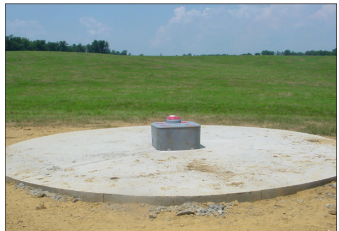
Figure 6. Circular concrete platforms provide a viable alternative to square concrete platforms. Note that the bare soil is due to construction. Photo by the Natural Resources Conservation Service of Kentucky.
