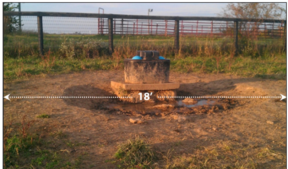
Figure 1. Without an all-weather surface, the HUA has eroded to the point where the watering facility is almost inaccessible and is no longer frost-proof. The depression also poses a threat to livestock health because livestock have to stand in mud and excrement to drink. Note the diameter of the bare soil area (18'). Photo by Jeff Lehmkuhler.
