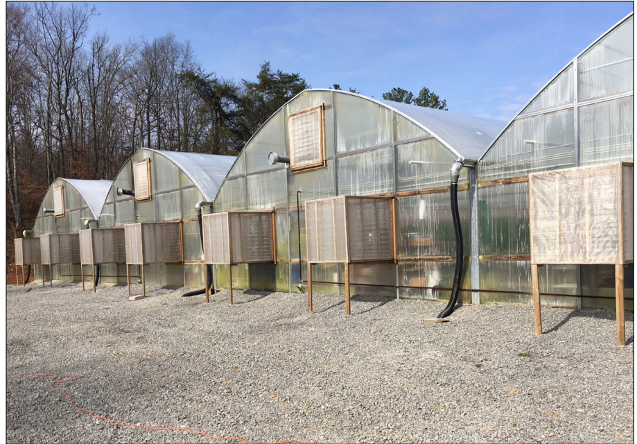
Insect screening over greenhouse openings and gravel around exterior.
