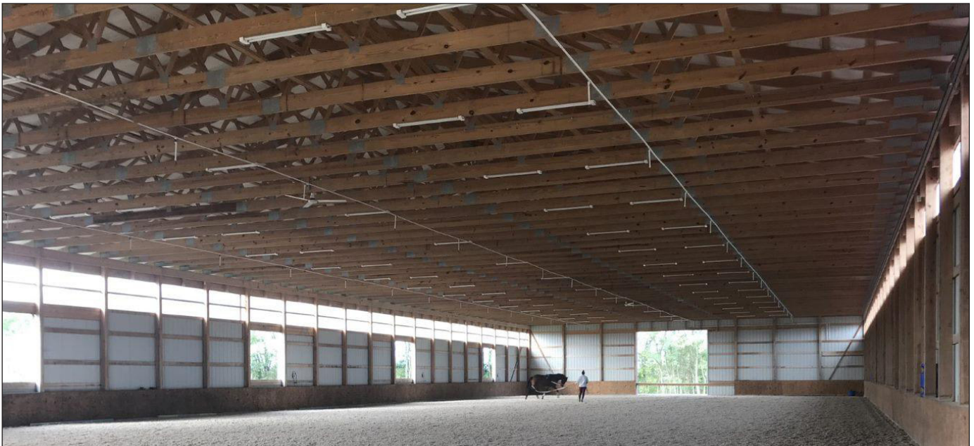
Figure 30. Overhead sprinkler system.
