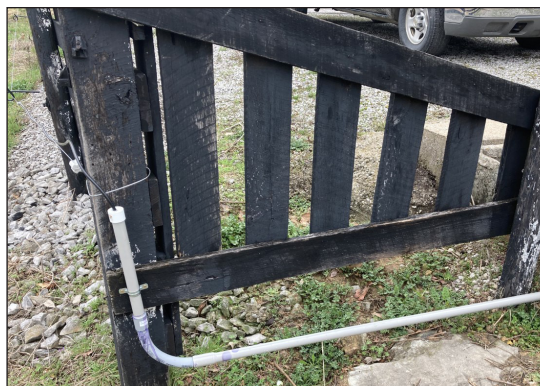
Figure 8. Double-insulated lead out wires going under gates should always be placed in a PVC pipe to protect the double insulated wire from breaks.
