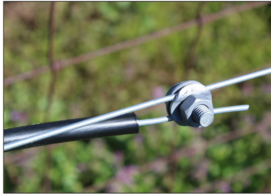
Figure 9. Make all connections using a high-quality, galvanized clamp or crimp. Wrapping wires results in loose connections which results in voltage losses.
