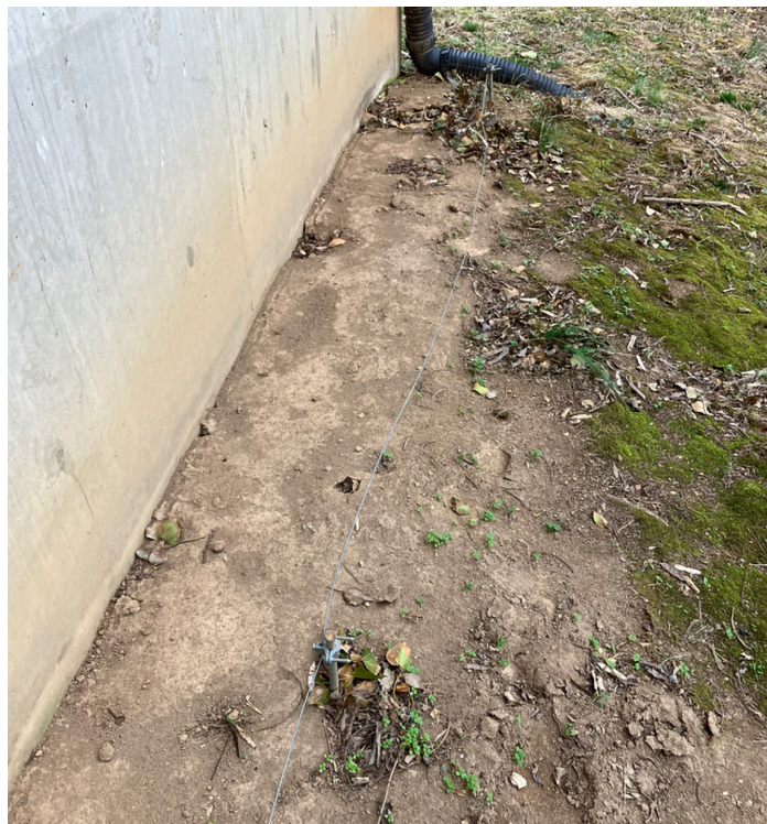
Figure 1. A series of ground rods are placed 10 feet apart along the north side of a barn.
