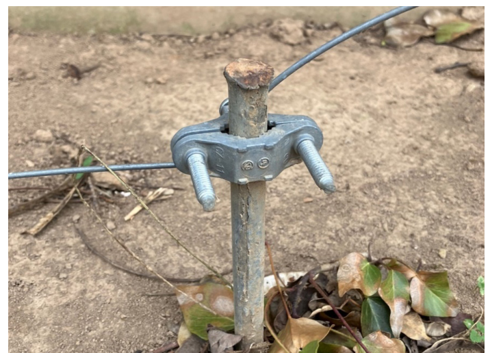
Figure 2. This galvanized ground rod is a good example of using like metal for the wire, clamp, and ground rod.
