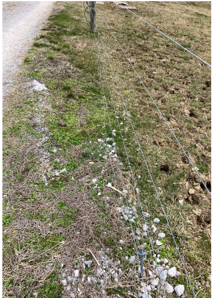
Figure 4. A ground system placed in a fence line is susceptible to damage from weed eaters, mowers, and other traffic. These systems should be checked regularly for continuity in the wire and good connections to the ground rods.
