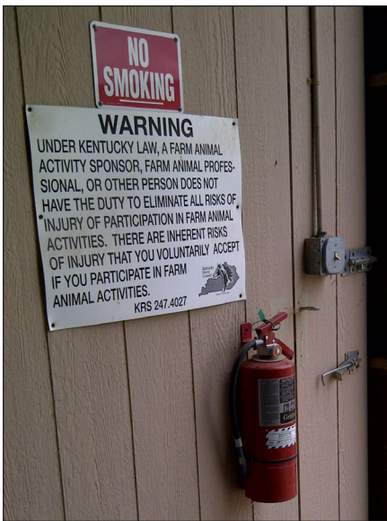
Fire extinguishers should be properly maintained and annually tested.
