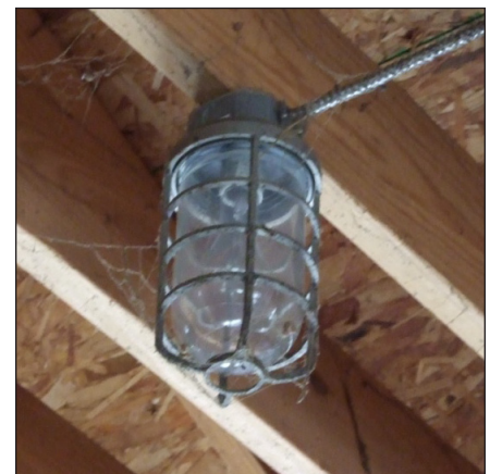
Light bulbs should be caged to prevent fire.
