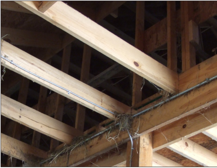
If possible, do not store hay in the barn loft. It makes cleaning more difficult and provides excellent fuel for spreading fires.
